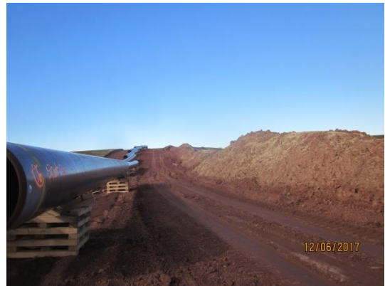
Strung pipe between Lancaster County Line and SR 0241. Stockpile lacks temporary stabilization.
