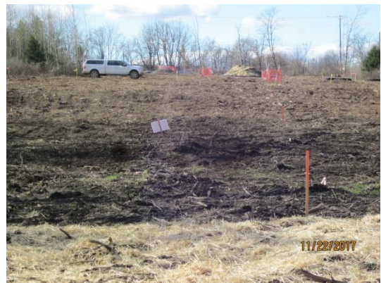
Quittapahilla creek ROW facing south. Lack of temporary stabilization.
