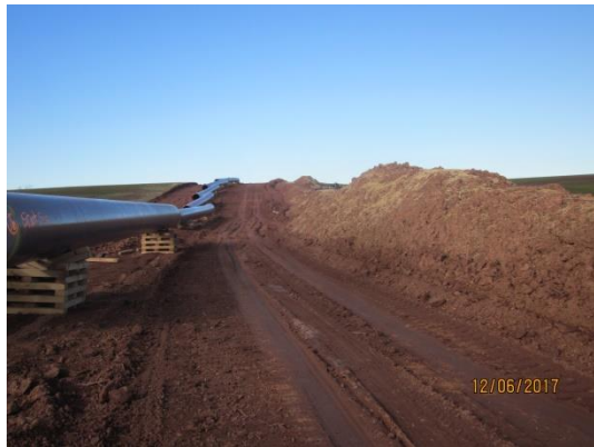
Strung pipe between Lancaster County Line and SR 0241. Stockpile lacks temporary stabilization.
