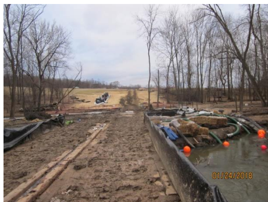
Mud covered bridge viewed from south side of creek.
