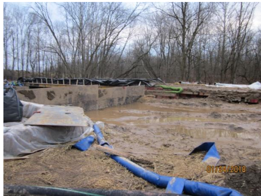
Steel plates on south side of creek keeping mud from entering creek.
