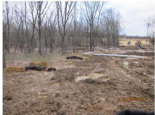
Mud in ROW on south side of creek. ECD's in place. Creek flow near top of bank.
