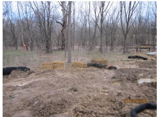
Sediment deposition off ROW in low lying area on south side of creek.
