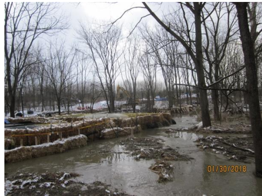
Pump water filter bag facilities discharging to low lying area on south side of stream.
