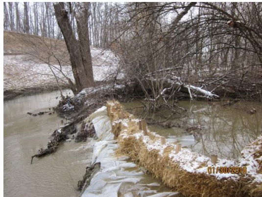
Straw bale dam near Clear Spring Road bridge. Sediment laden water entering stream.
