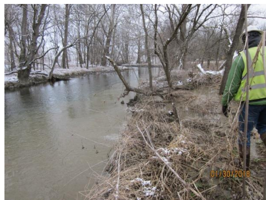
Sediment laden water entering stream after passing through pump water filter bag facility.
