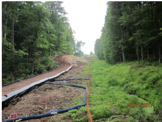
West of Beech Street sock installed, slope seeded and mulched with straw
