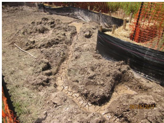
Area of frac-out. Drilling mud removed. Conveyance to vac pit and vac pit visible in photo.
