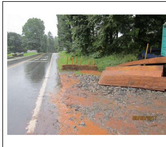
Small trail of sediment laden runoff visible leaving rce on east side of SR 0017
