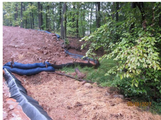
Overtopped filter sock on west side of SR 0117 in area of waterbody crossing S A 14.
