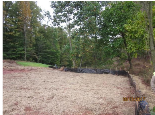
Back toward beech street. View downstream toward first timber bridge (S-A1). Suggest installation of sediment trapping facility in area of outside corner of silt fence.
