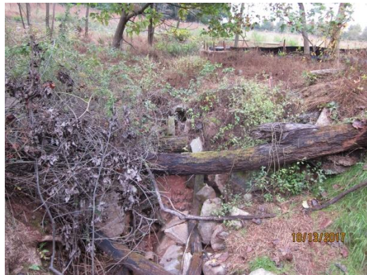
View from timber bridge (S-A1) looking upstream. Sediment deposition in debris pile near bottom center of photo and in area of silt fence and straw bales in upper right portion of photo.
