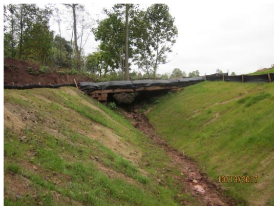
View looking upstream (S-A1) under first timber bridge west of beech street.
