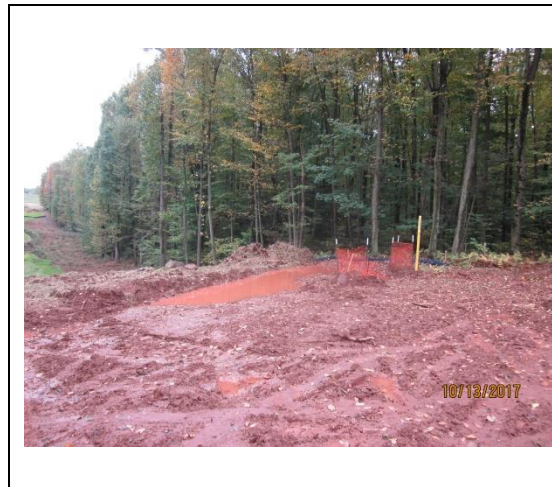
Water bar and sock filter/sump west of crossing S-A3 in area west of beech street .
