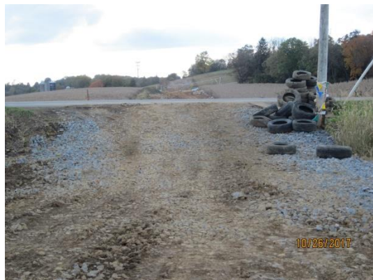
RCE east side of Cornwall Road requires maintenance.
