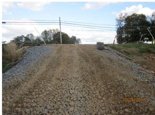
RCE on west side of Cornwall road requires maintenance.
