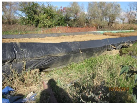
Geotextile under timber bridges (S-A25 and P-A1-A and P-A1-B) stressed and bulging with excess sediment and/or unmaintained.
