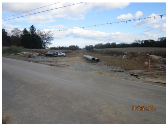
RCE on east side of Tice Lane requires maintenance.
