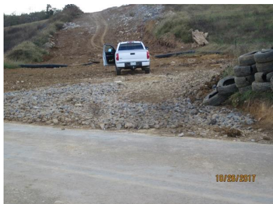
RCE on west side of Tice Lane requires maintenance.
