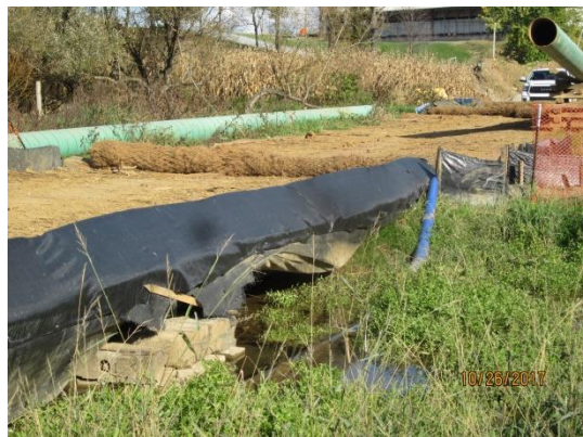
Geotextile under timber bridges (S-A25 and P-A1-A and P-A1-B) stressed and bulging with excess sediment and/or unmaintained.
