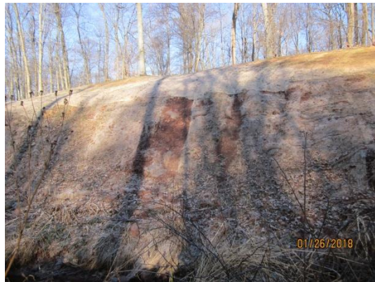
Slight slump in area of Killinger Creek, west of Beech Street.
