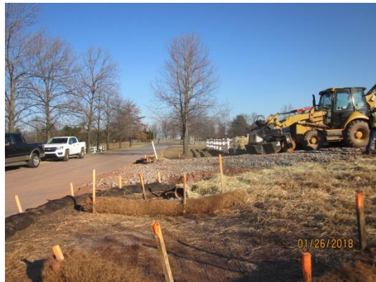
Recently installed culvert pipe, RCE and ECD's on east side of Beech Street.
