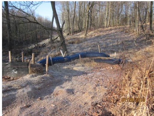
Sock trap/J-hook in area upslope of S-A3. Debris trail suggests runoff went around right side of sock.
