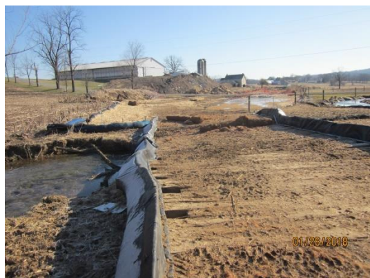
Upper left portion of timber bridge slightly sunken. Bridge located west of Ridge Lane.
